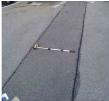
Figure 33 Low Patch PAVERTM Distress Identification Manual
