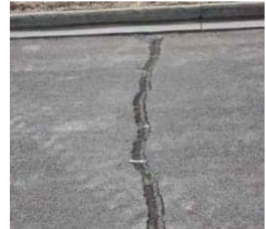
Figure 20 High T&L Cracking PAVER™ Distress Identification Manual
