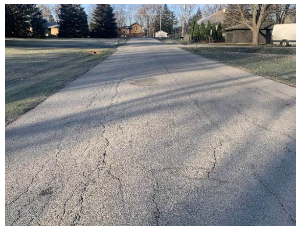
Figure 41 Fair Roadway Condition Apple Avenue
