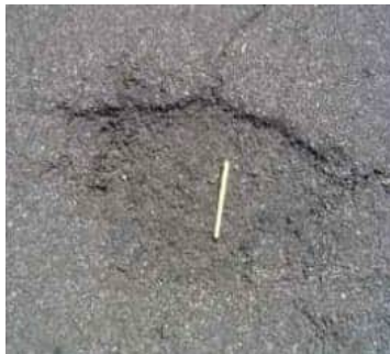
Figure 30 Low Pothole PAVER™ Distress Identification Manual
