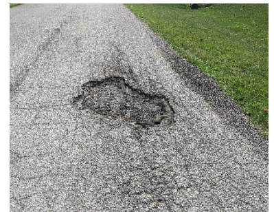
Figure 46 Pothole on Saddlebrook Lane
