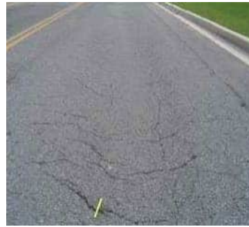
Figure 13 Medium Slippage PAVER™ Distress Identification Manual
