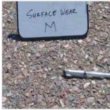
Figure 4 Medium Weathering PAVER™ Distress Identification Manual
