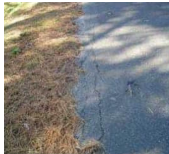
Figure 28 Medium Edge Cracking PAVERTM Distress Identification Manual
