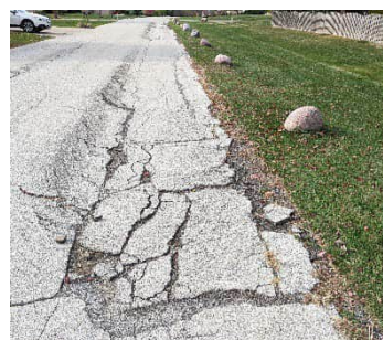
Figure 45 High Slippage Cracks on West Briar Patch Lane
