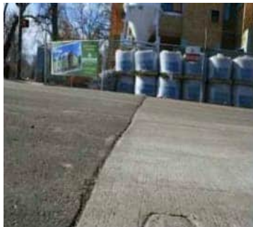
Figure 9 Low Shoving PAVER™ Distress Identification Manual
