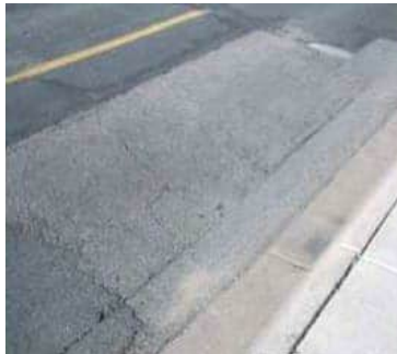
Figure 34 Medium Patch PAVERTM Distress Identification Manual
