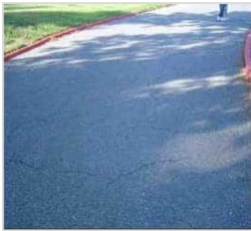
Figure 21 Low Block Cracking PAVER™ Distress Identification Manual
