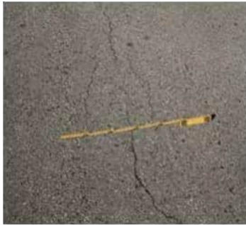
Figure 24 Low Alligator Cracking PAVERTM Distress Identification Manual
