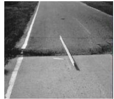
Figure 11 High Shoving PAVER™ Distress Identification Manual
