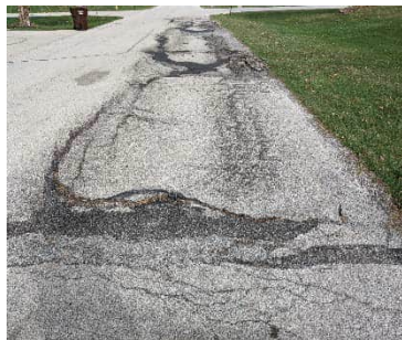
Figure 44 High Slippage Cracks on East Red Coat Drive
