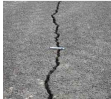
Figure 19 Medium T&L Cracking PAVER™ Distress Identification Manual
