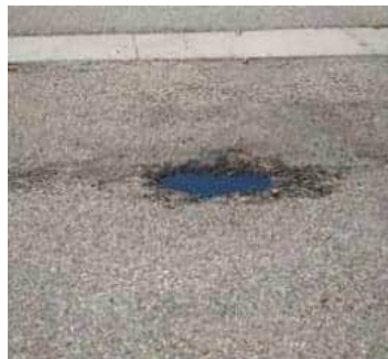
Figure 31 Medium Pothole PAVER™ Distress Identification Manual
