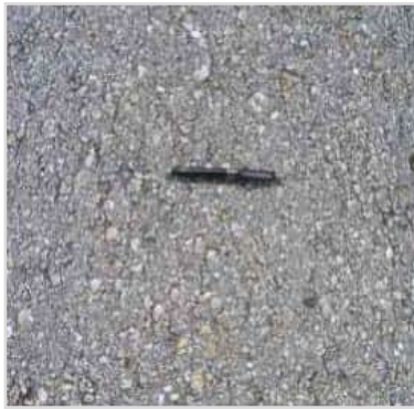
Figure 3 Low Weathering PAVER™ Distress Identification Manual
