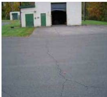
Figure 18 Low T&L Cracking PAVER™ Distress Identification Manual
