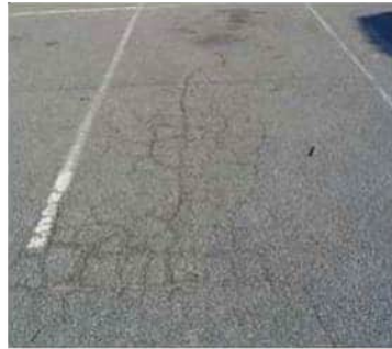
Figure 25 Medium Alligator Cracking PAVERTM Distress Identification Manual
