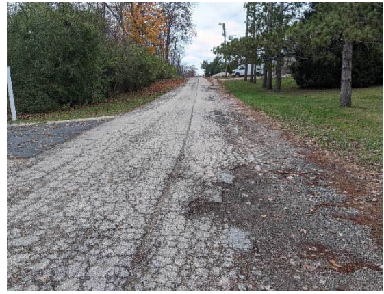
Figure 43 Serious Roadway Condition 135th Street
