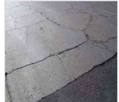
Figure 23 High Block Cracking PAVER™ Distress Identification Manual
