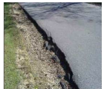
Figure 38 High Drop-Off PAVERTM Distress Identification Manual
