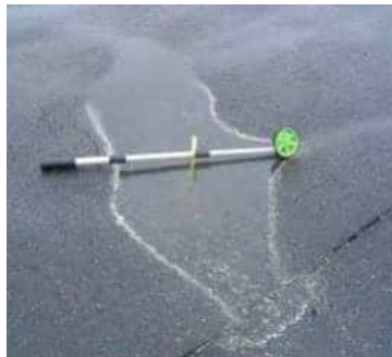
Figure 16 Medium Depression PAVER™ Distress Identification Manual
