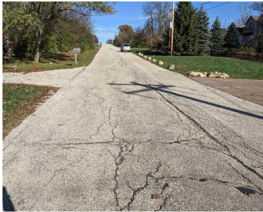
Figure 42 Poor Roadway Condition Gordon Lane
