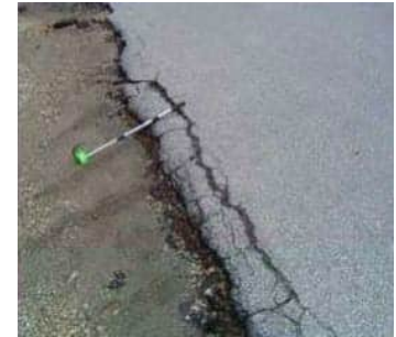
Figure 29 High Edge Cracking PAVERTM Distress Identification Manual
