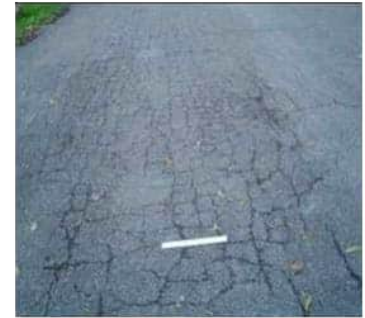
Figure 26 High Alligator Cracking PAVERTM Distress Identification Manual
