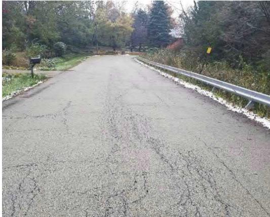
Figure 42 Poor Roadway Condition Gordon Lane (Middle), Lemont, Illinois
