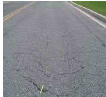
Figure 13 Medium Slippage PAVER™ Distress Identification Manual
