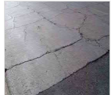
Figure 23 High Block Cracking PAVER™ Distress Identification Manual
