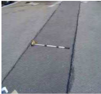
Figure 33 Low Patch PAVERTM Distress Identification Manual
