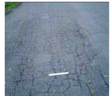
Figure 26 High Alligator Cracking PAVERTM Distress Identification Manual
