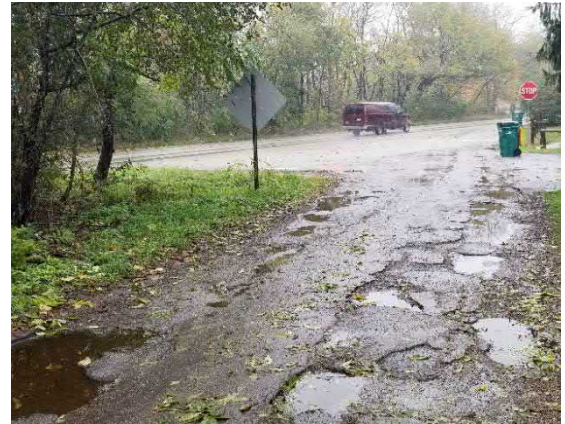
Figure 43 Serious Roadway Condition Kotlin Road, Lemont, Illinois
