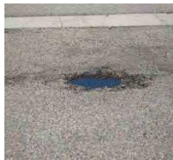
Figure 31 Medium Pothole PAVER™ Distress Identification Manual
