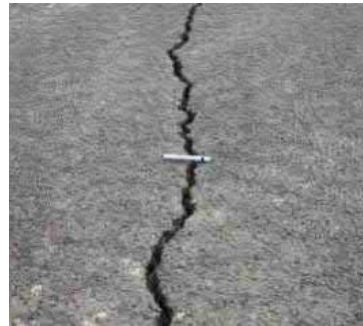
Figure 19 Medium T&L Cracking PAVER™ Distress Identification Manual
