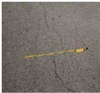
Figure 24 Low Alligator Cracking PAVERTM Distress Identification Manual
