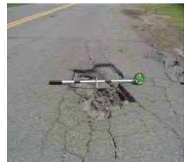
Figure 32 High Pothole PAVER™ Distress Identification Manual
