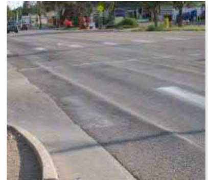
Figure 8 High Rutting PAVER™ Distress Identification Manual
