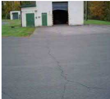
Figure 18 Low T&L Cracking PAVER™ Distress Identification Manual
