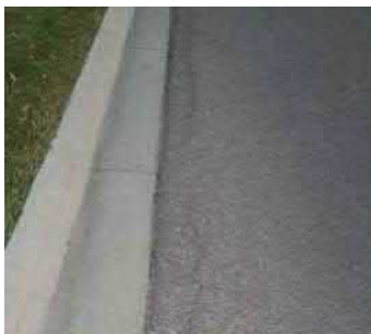
Figure 27 Low Edge Cracking PAVERTM Distress Identification Manual
