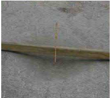
Figure 17 High Depression PAVER™ Distress Identification Manual
