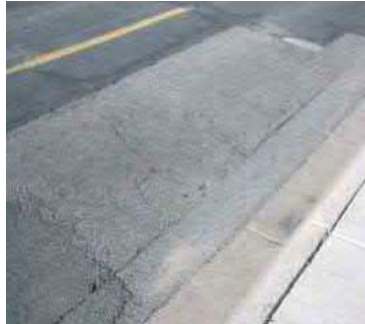
Figure 34 Medium Patch PAVERTM Distress Identification Manual
