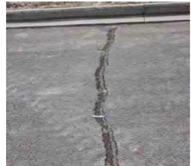
Figure 20 High T&L Cracking PAVER™ Distress Identification Manual
