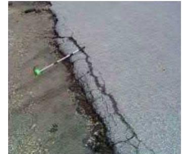
Figure 29 High Edge Cracking PAVERTM Distress Identification Manual
