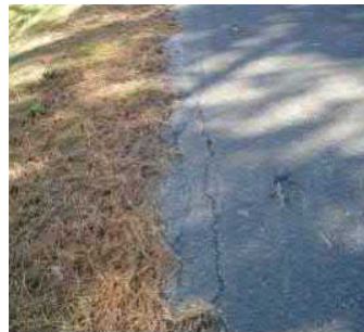
Figure 28 Medium Edge Cracking PAVERTM Distress Identification Manual
