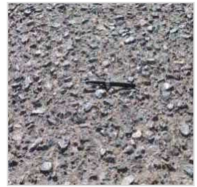
Figure 5 High Weathering PAVER™ Distress Identification
