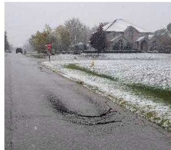
Figure 45 High Slippage Cracks on East Red Coat Drive
