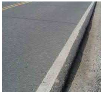
Figure 37 Medium Drop-Off PAVERTM Distress Identification Manual
