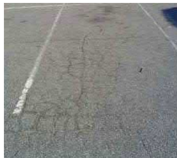
Figure 25 Medium Alligator Cracking PAVERTM Distress Identification Manual
