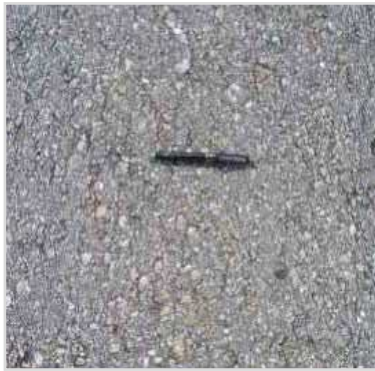
Figure 3 Low Weathering PAVER™ Distress Identification Manual
