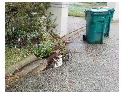
Figure 46 Pavement Cave-in on Fox Lane
